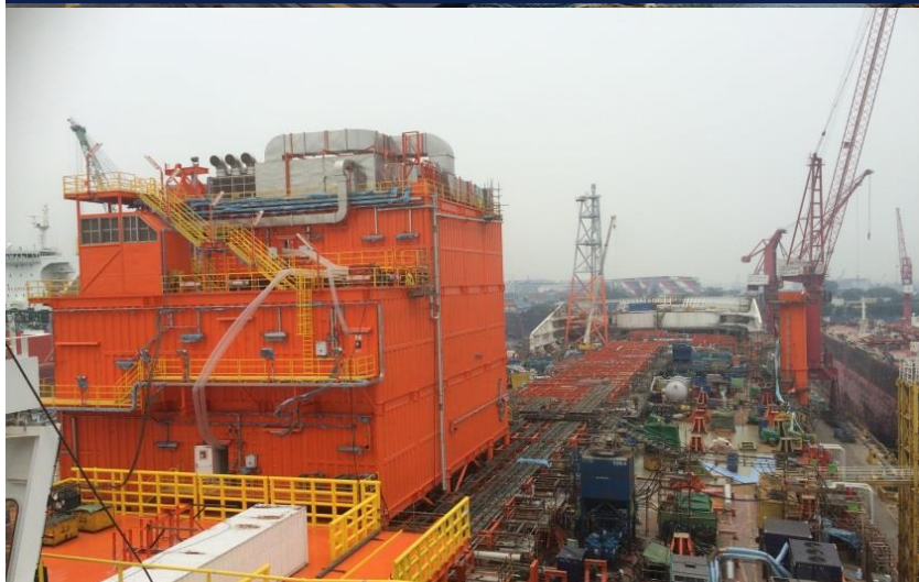
E-House & laydown installed on main deck
