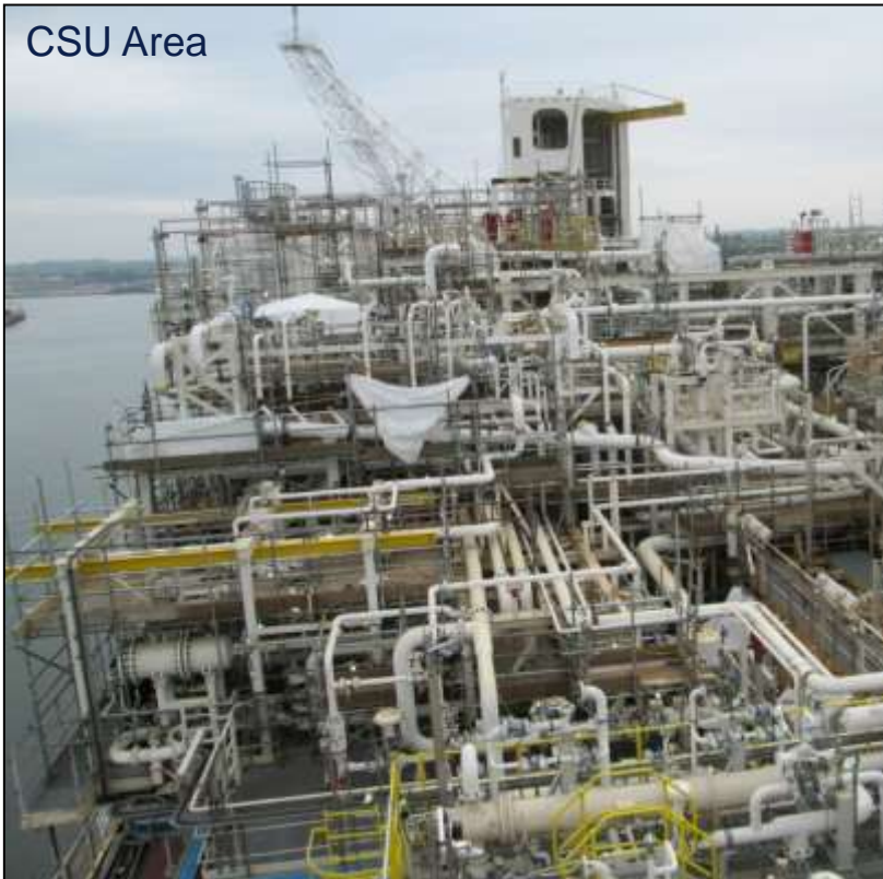
Water Injection Aft
